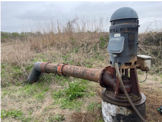
Electric turbine relift
