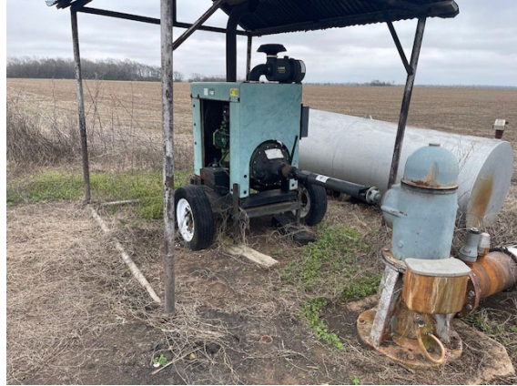
One of two diesel turbine wells
