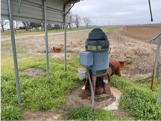
One of three electric turbine wells
